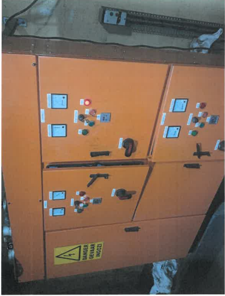
Figure 1: New Ventures Pump Station Switchgear Panel
