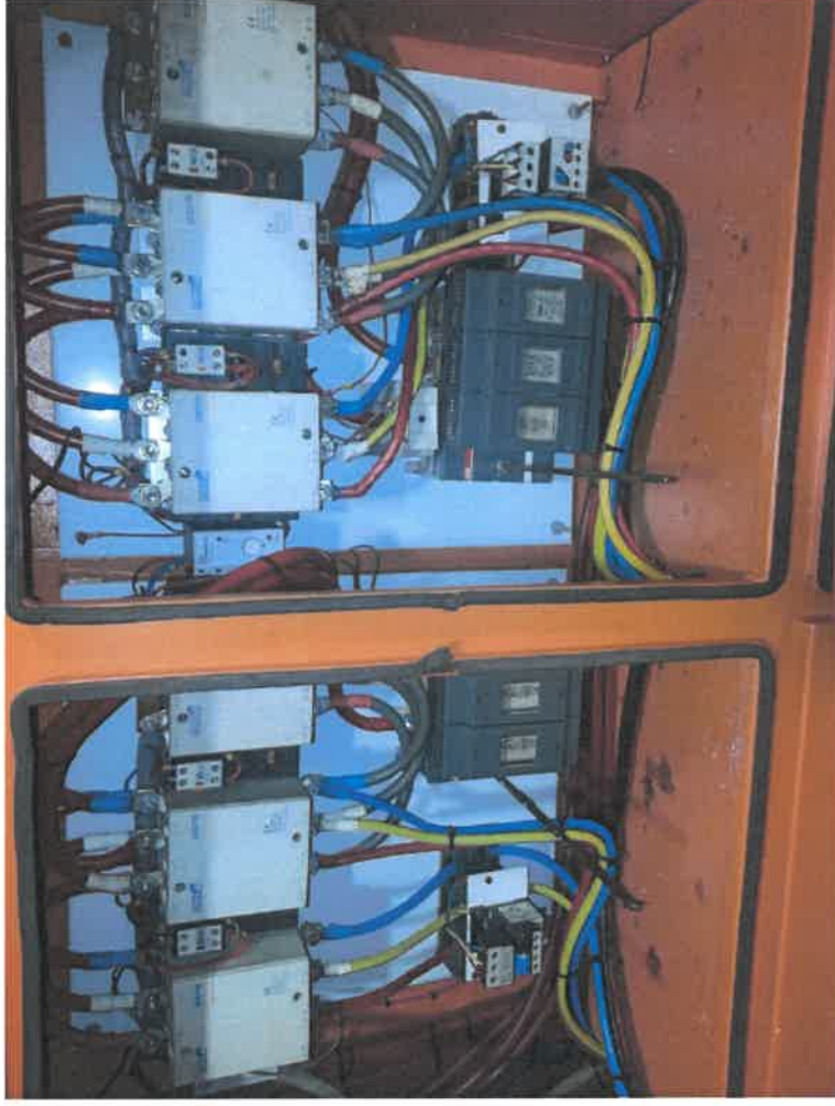
Figure 2: Switchgear panel (Pump 1 and 2)
