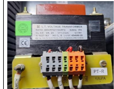
BOQ 18: Voltage Transformer
